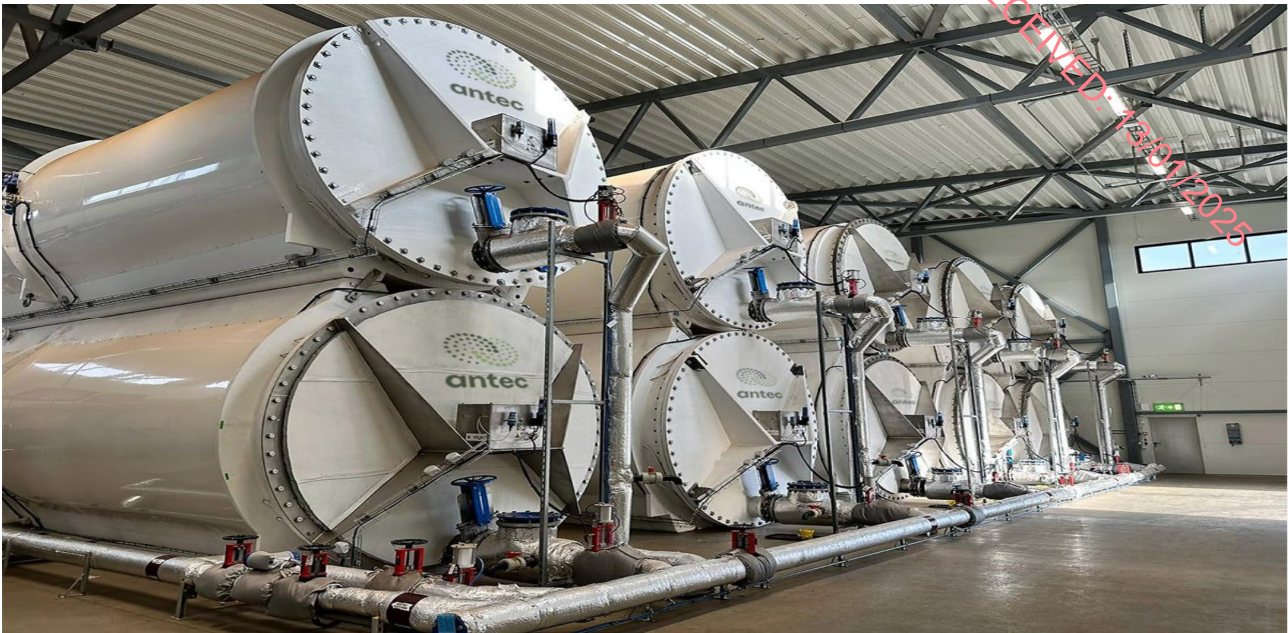
Plate 2-3: Typical Reactor Bank
